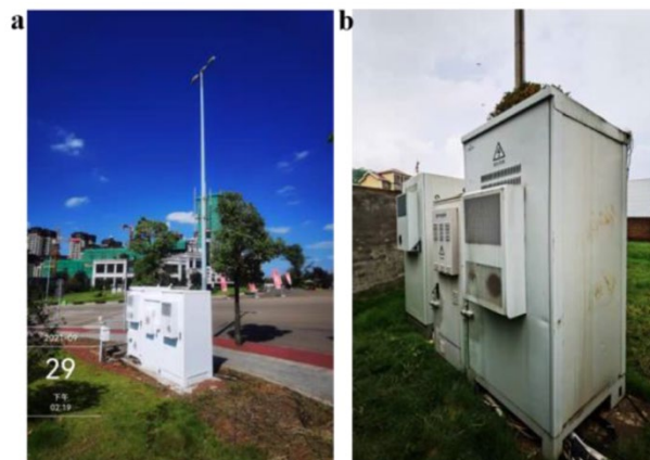
Figure 8 - Photos of the 4G Base Stations (a) with and (b) Without a Superamphiphobic Self-Cleaning PSDRC Coating Located in Ziyang, Sichuan Province, China. [16]
