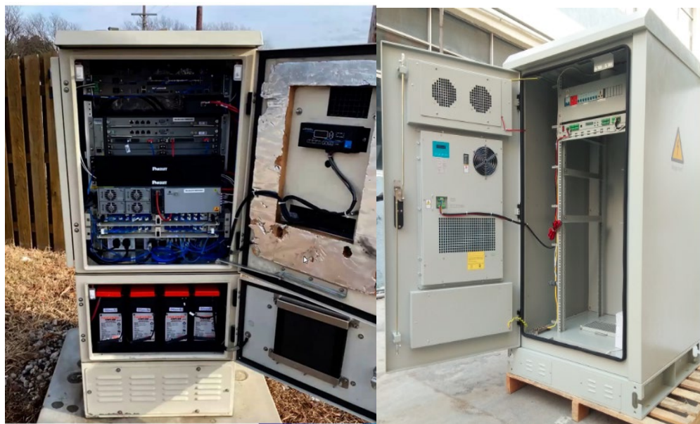
Figure 1- Sample of Telecommunication Outside Plant Cabinet [1][4]
