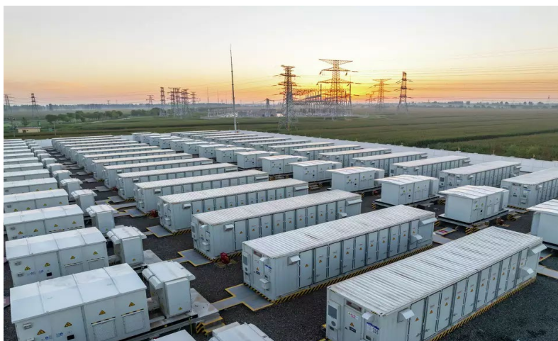
Figure 8 - Battery Storage for Grid in Arizona
